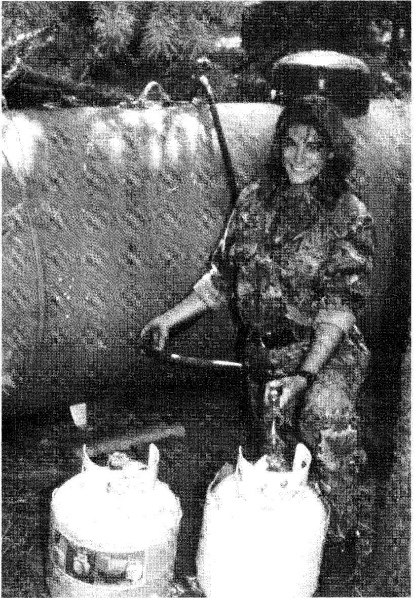
Small 5-gallon LP gas tanks can be filled from a large nurse tank if proper equipment is installed before the main tank is first filled.
