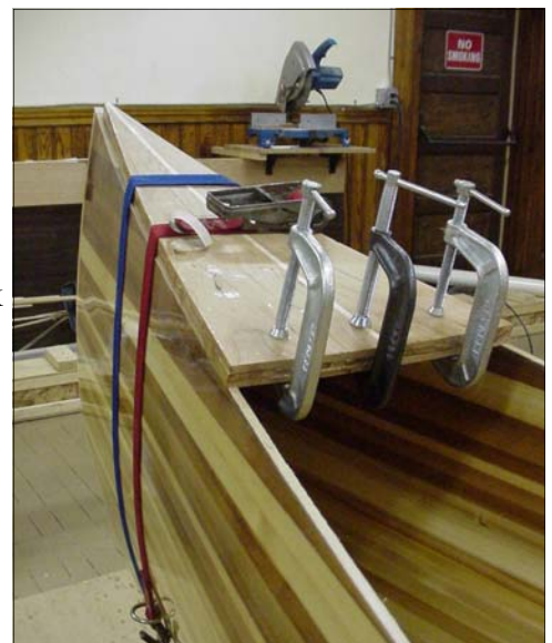
This shows the deck being glued to match the curve of the sheerline. When cured it will be cut to fit inside the inwales. This glue up can be done when the sheerline is cut (as shown here) OR later after the inwales are installed.
