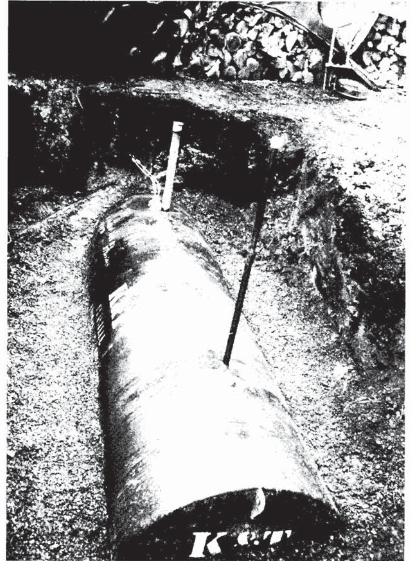
This fiberglass-coated underground oil tank will last without maintenance for 50 years or more, providing an unseen source of energy for the retreat. Note the firewood in the background—this retreator has many contingency plans.
